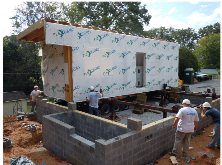
Figure 1. The first modular unit is set onto rollers before being shifted laterally across the staged foundation wall.
